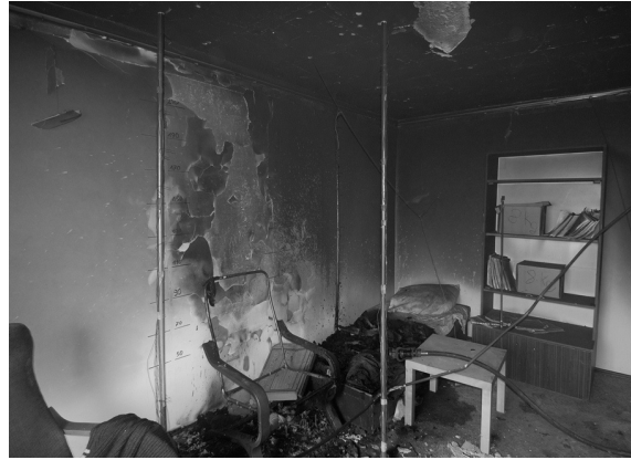
Fig. 4 Fire compartment after test no.1
