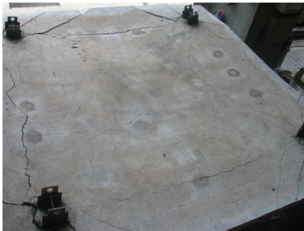
Fig. 6 Crack pattern of S2-FR-IB
