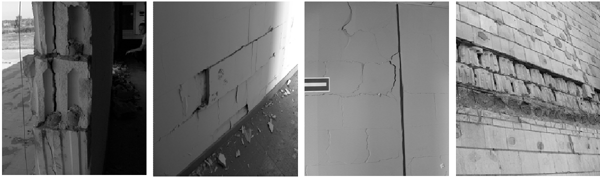
Fig. 3 Examples of the structural damage to the wall
